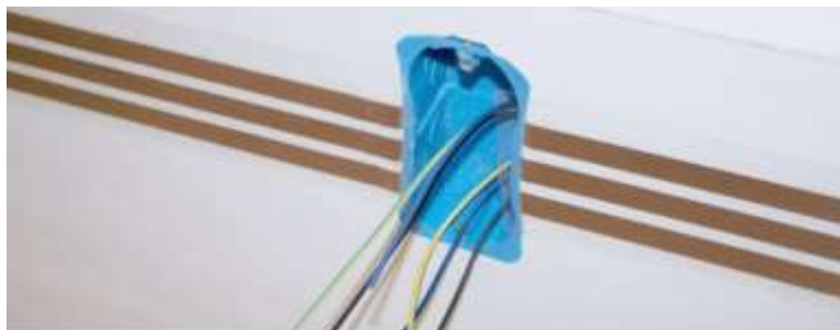
Figure 15: Example: integration of a light fixture from controlled light socket using flat tape. The integration is minimally invasive, quickly executed, and environmentally effective, with all the advantages mentioned.
