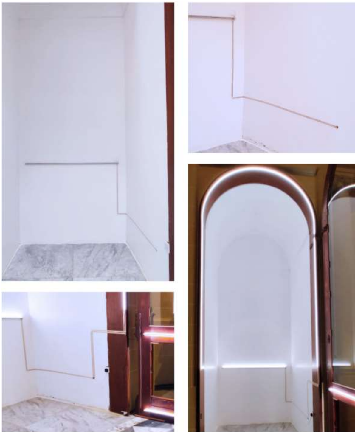
Figure 20: Implementation of a lighting system for a statue placed in a niche in the church with Electrical Tapes NM2BT05 and NM2BT15 and Next-Light LEDs
