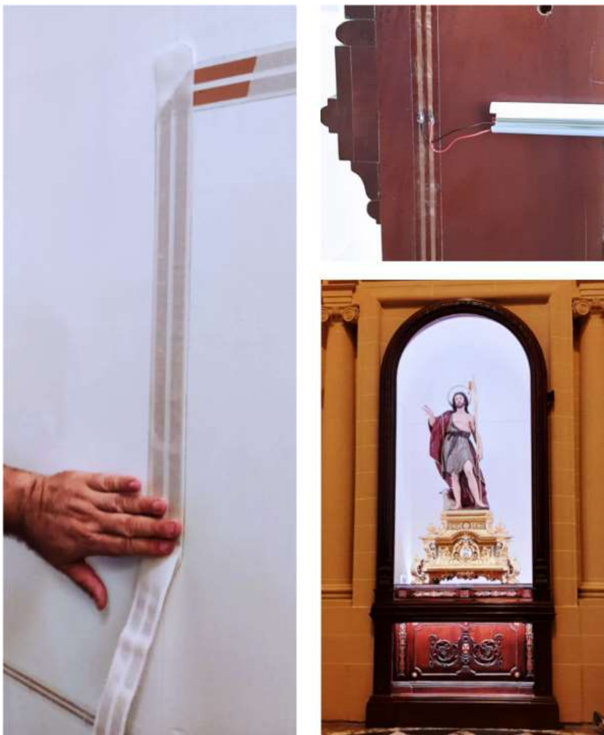
Figure 21: Implementation of a lighting system for a statue placed in a niche in the church with Electrical Tapes NM2BT05 and NM2BT15 and Next-Light LEDs
